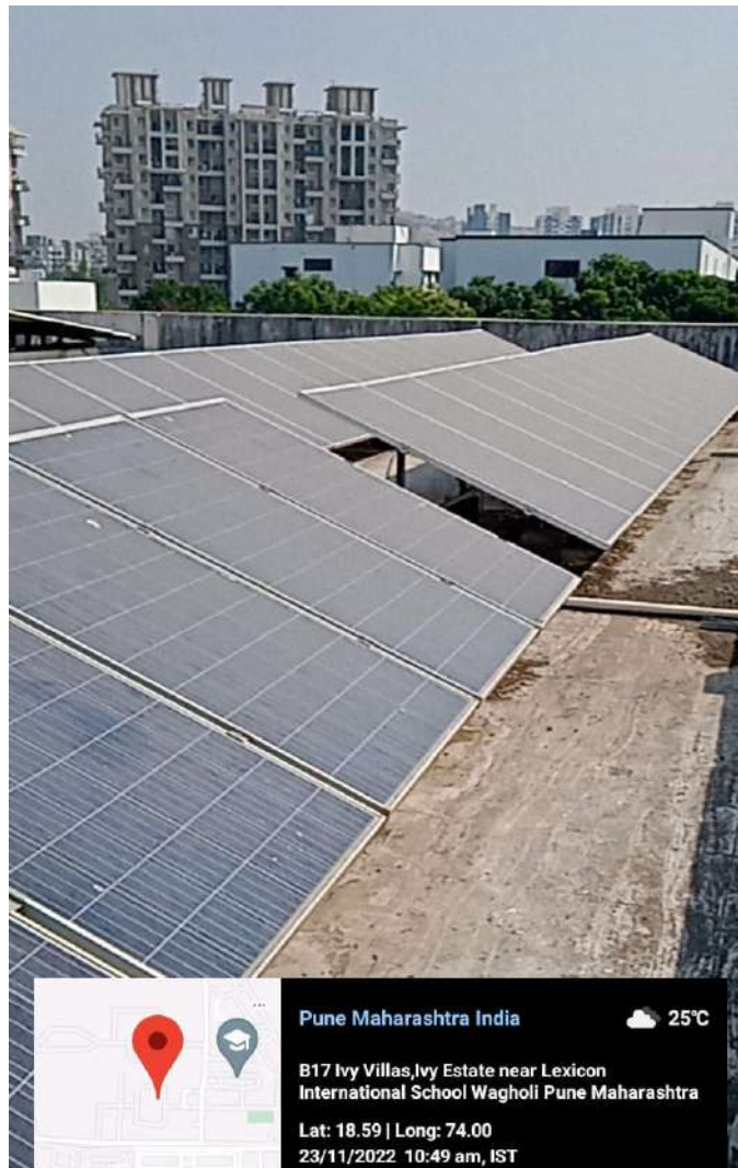
Fig. 1 Solar panle on roof of building-C
