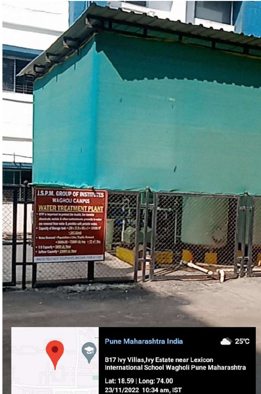
Fig. Water Treatment Plant at at ICOER
